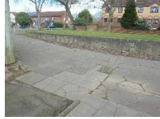
Uneven/broken pavement slabs
